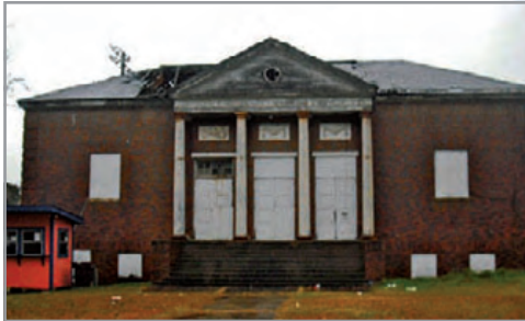
Marion Elementary School, Marion, Loan for Emergency Repairs
