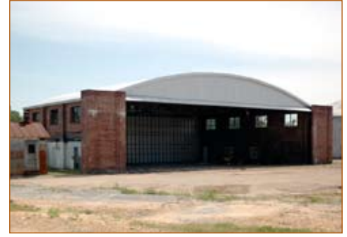
W.P.A. Hangar, Gragg-Wade Field, Clanton, Chilton County; Note that the hangar doors are yet to be installed.
